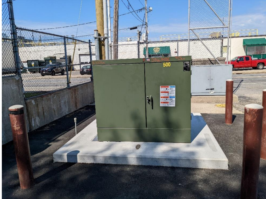
Figure 9 Dedicated Transformer for BEB Chargers at 114 Valley St
